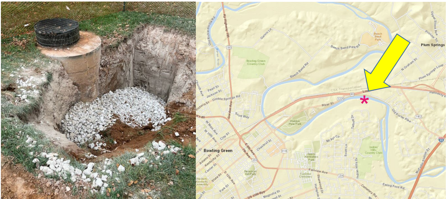
Figure 4- Operations crews and the City Geologist repaired a sinkhole near McClintock Ct (4-6 November)
