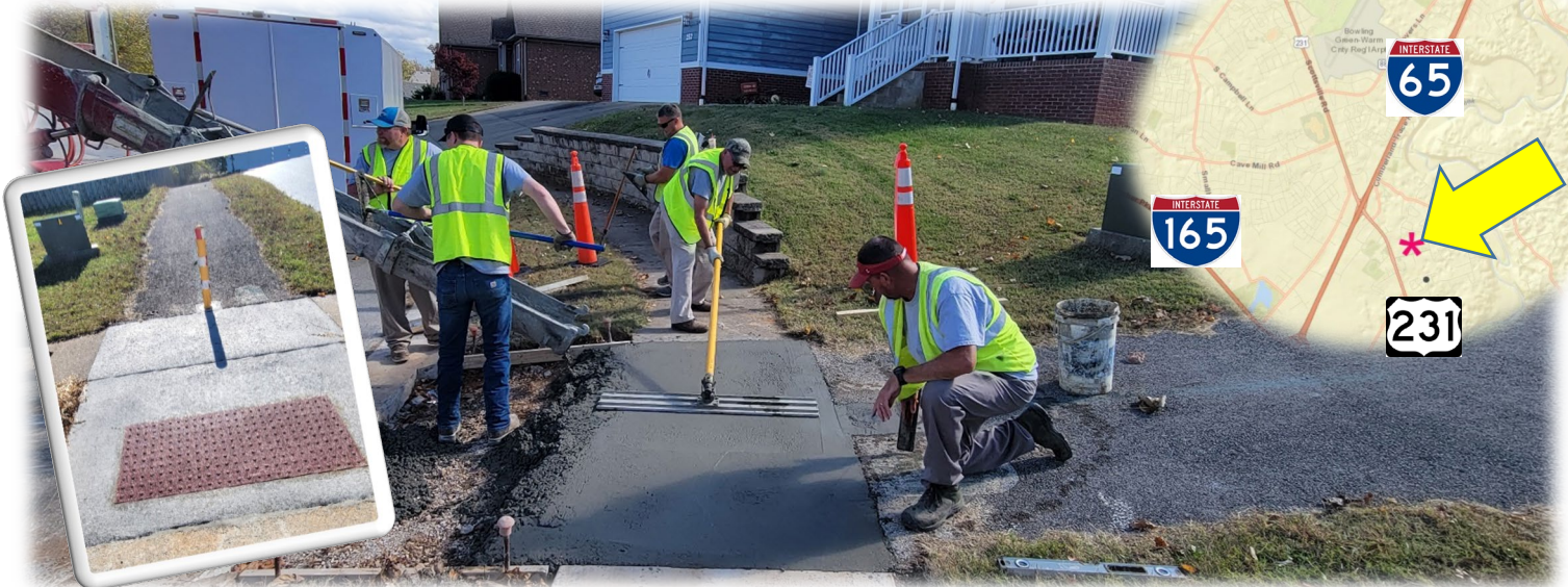
Figure 2- The cement crew poured a new ADA compliant ramp and installed a new bollard at the Atlanta Way greenway entrance (5 November)
