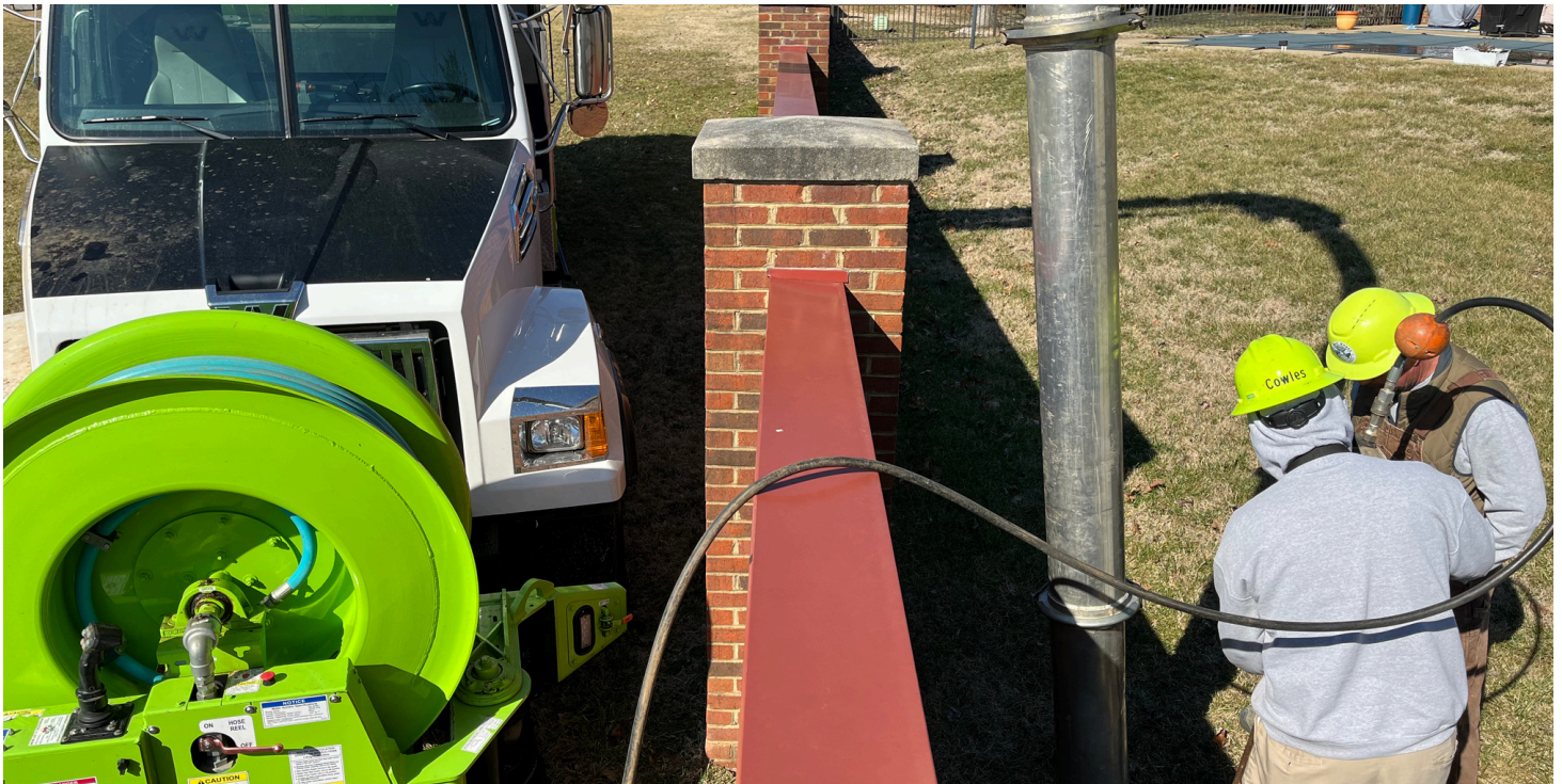
Operations Maintenance Technician II Timmy Cowles leads a team hydroexcavating a sinkhole near St. Andrews Circle. Water was used due to the proximity of exposed utility lines (10 February).
