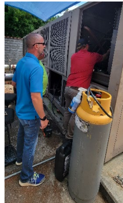
Figure 9- Facilities Manager Dave Hehner oversees air conditioner compressor repair work at the Convention Center (15 August)
