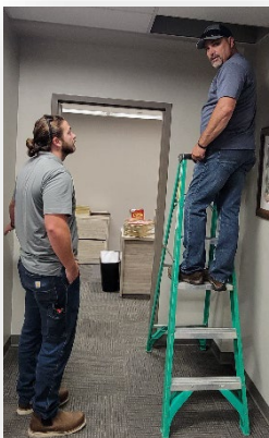
Figure 8- Facilities Maintenance Technicians Caleb Houtchen (left) and Kenny Woods (right) move conduit at the NCS building (14 August)
