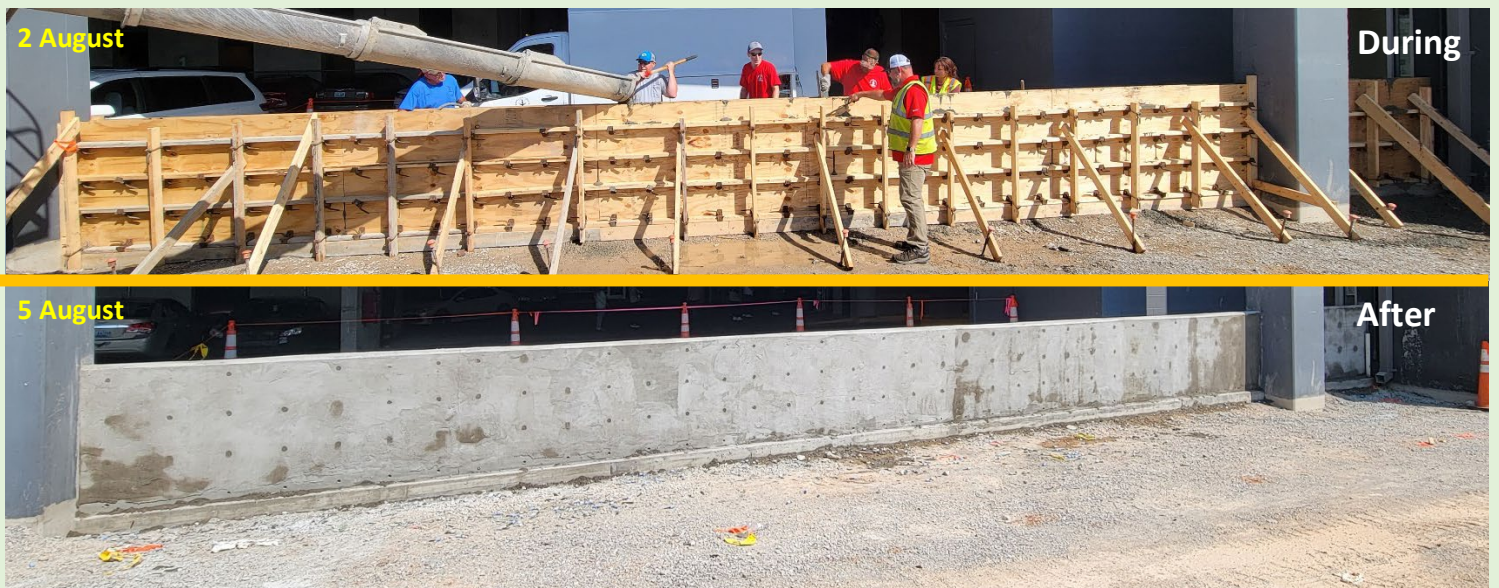
Figure 1- Our Operations Concrete team constructed a wall at the College Street Parking Garage to support the development of the space into a food truck rally point and picnic area called The Fringe (2-6 August)
