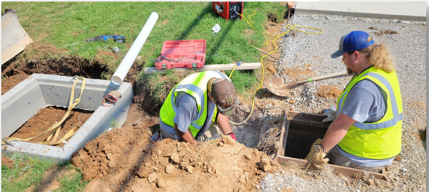
Figure 2- Operations Maintenance Technician II Timmy Cowles (Left) and Operations Maintenance Technician III Matt White (Right) install a new stormwater drain along Gordon Ave as part of the new greenway (5 August)
