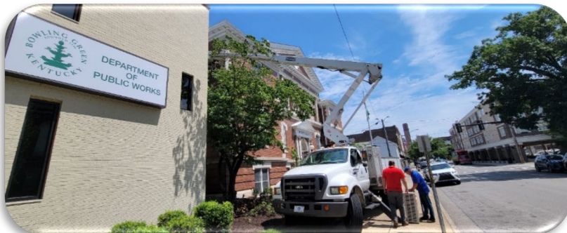
Figure 8- Facilities Technicians Kenny Woods and Caleb Houtchen assist with the replacement of an HVAC unit at City Hall (8 July)
