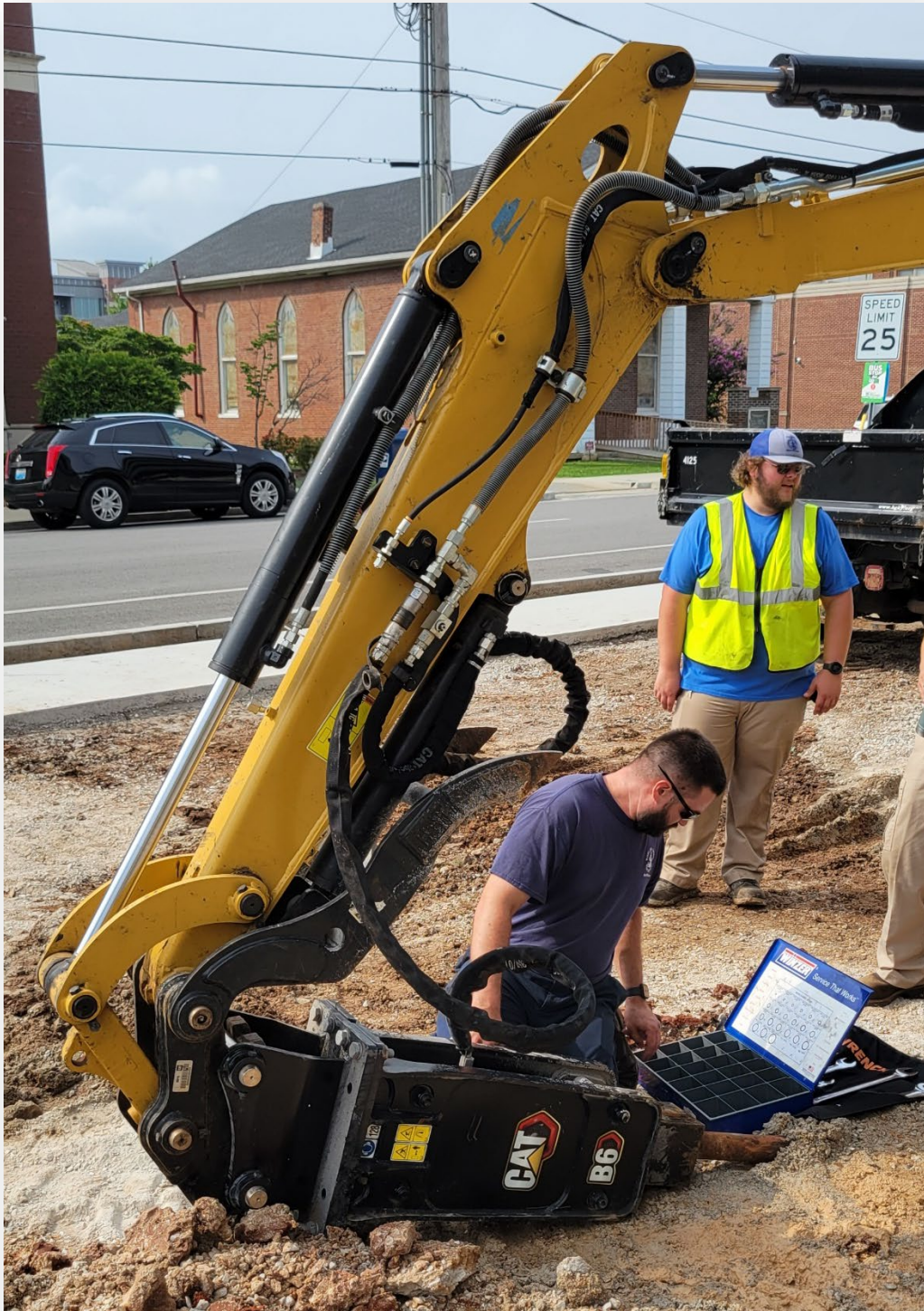
Figure 10-Master Technician Josh Johnson repairs a hydraulic line at the future site of The Fringe on College Street (23 July).
