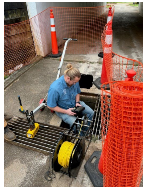
Figure 8-Environmental Compliance Coordinator Nick Lawhon drives a remote camera into a drainage pipe at CrossWinds Golf Course (8 April)
