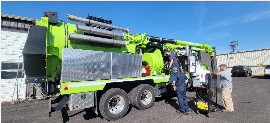
Figure 13-Immediate Work Order-Master Technician Josh Johnson and Service Technician Nick Updegraff repair a hydraulic line on the Vactor truck while Operations Maintenance Technician II Timmy Cowles waits. (23 April)
