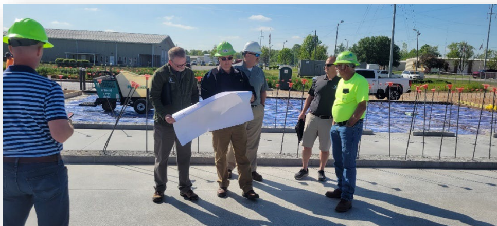
Figure 9-Facilities Manager Dave Hehner oversees construction coordination at Fire Station #5 on Porter Pike (24 April)
