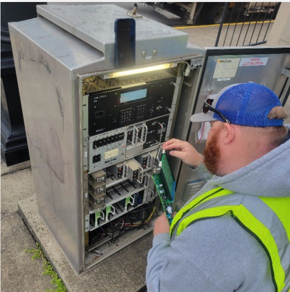
Figure 2- Signal Technician I Josh Minton repairs a signal box on State St & E. 12 th Ave (3 Apr)
