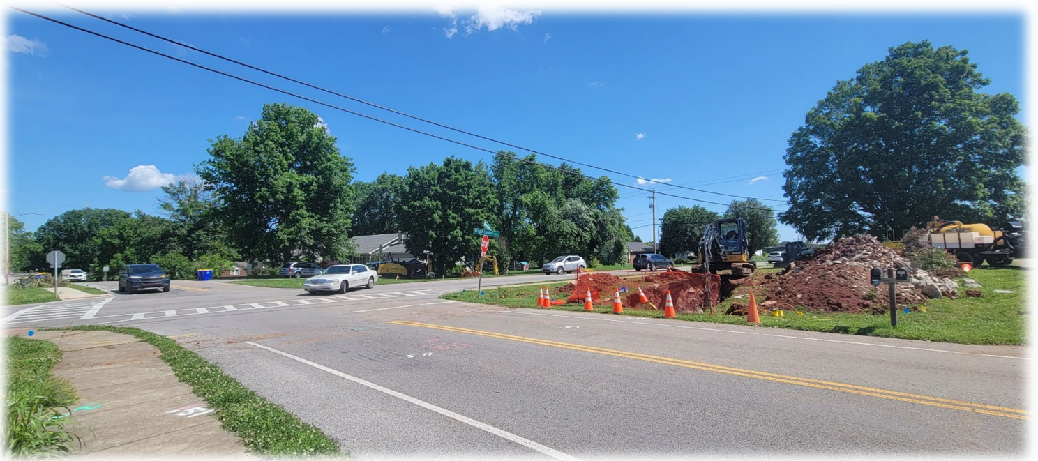
Figure 6- Construction has started on the last of 4 roundabouts on Westen Street. This final location will be on the corner of Westen Street and Highland Way. Construction should be completed before school starts in the fall. Roundabouts are already in place on Westen Street at Patrick Way, Rockingham Avenue and Ashley Circle. When completed, this will mark the 15th roundabout in the city. (29 May)
