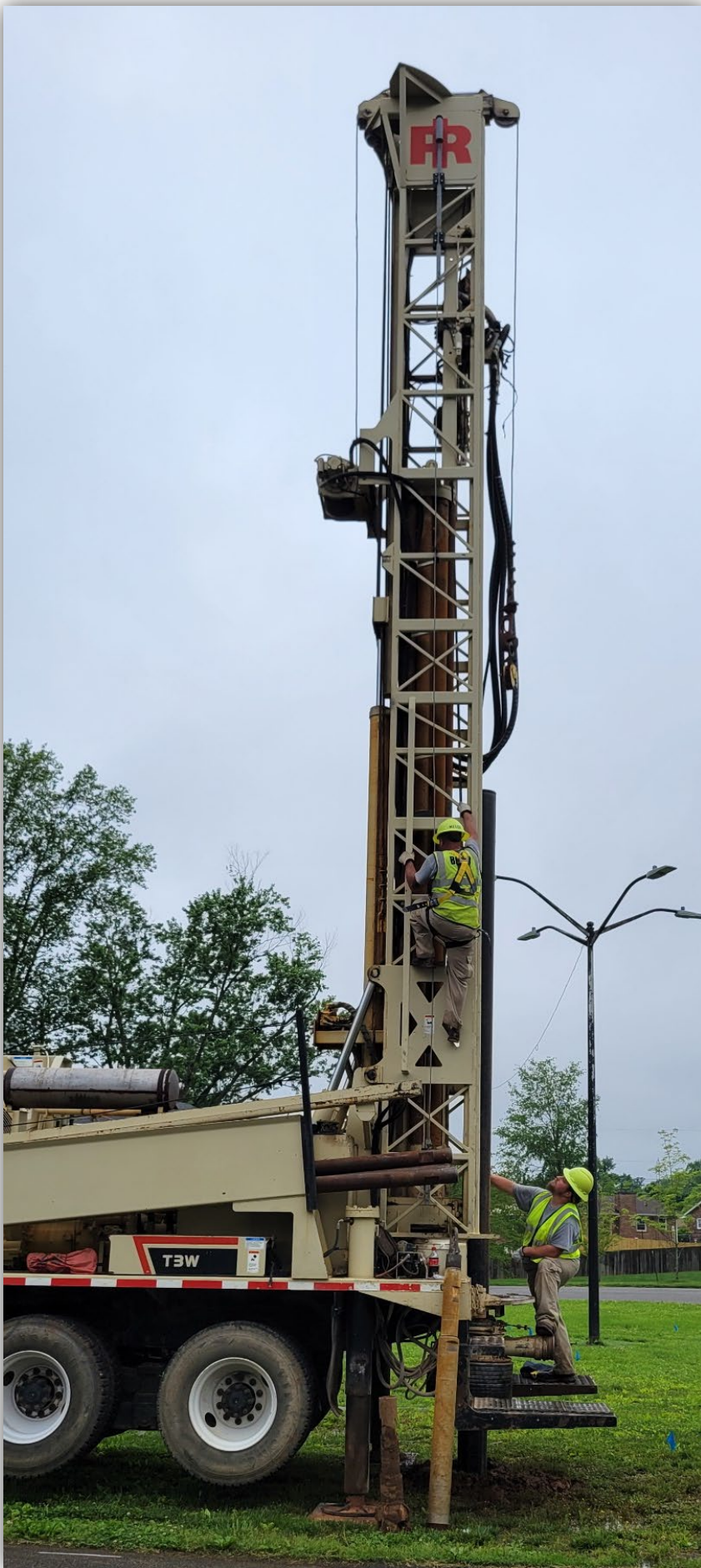
Figure 5- (left) Crew Leader Josh Miller (climbing) and Operations Maintenance Technician III Matt White (Below) work on the drill rig. It was being used to install a Class V injection well for stormwater on Spruce Court. The City of Bowling Green closely monitors the placement and maintenance of over 1,000 injection wells placed throughout the city. There are over 531,000 Class V wells across the United States. (15 May).
