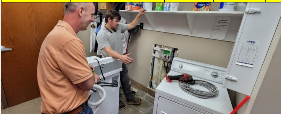
Figure 9- Facilities Manager Dave Hehner helped troubleshoot a plumbing issue at Fire Station #2 (Airport) on 15 May.
