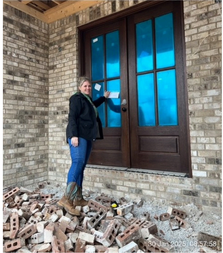
Construction Coordinator I Dara Price documents construction violations (30 January).
