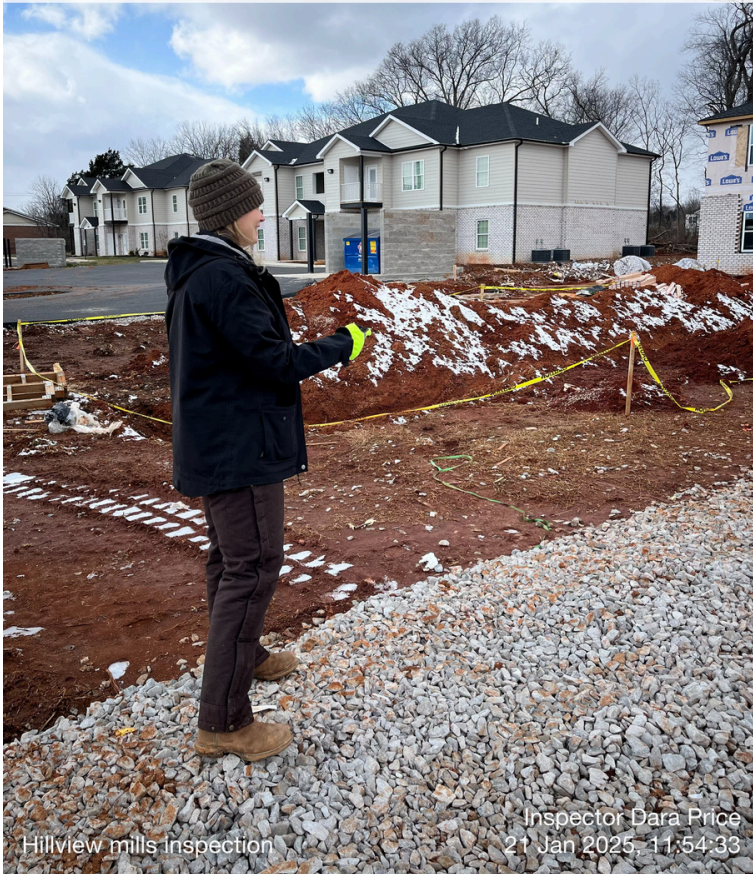
Construction Coordinator I Dara Price conducts an inspection at Hillview Mills (21 January)
