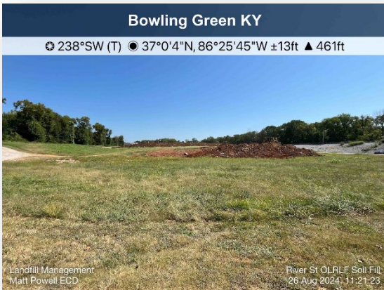
Figure 9- Work to fill low spots in the protective cap of the River St Landfill is scheduled for completion in October. Working for mutual benefit with a local contractor saved the City several hundred thousand dollars for the work.
