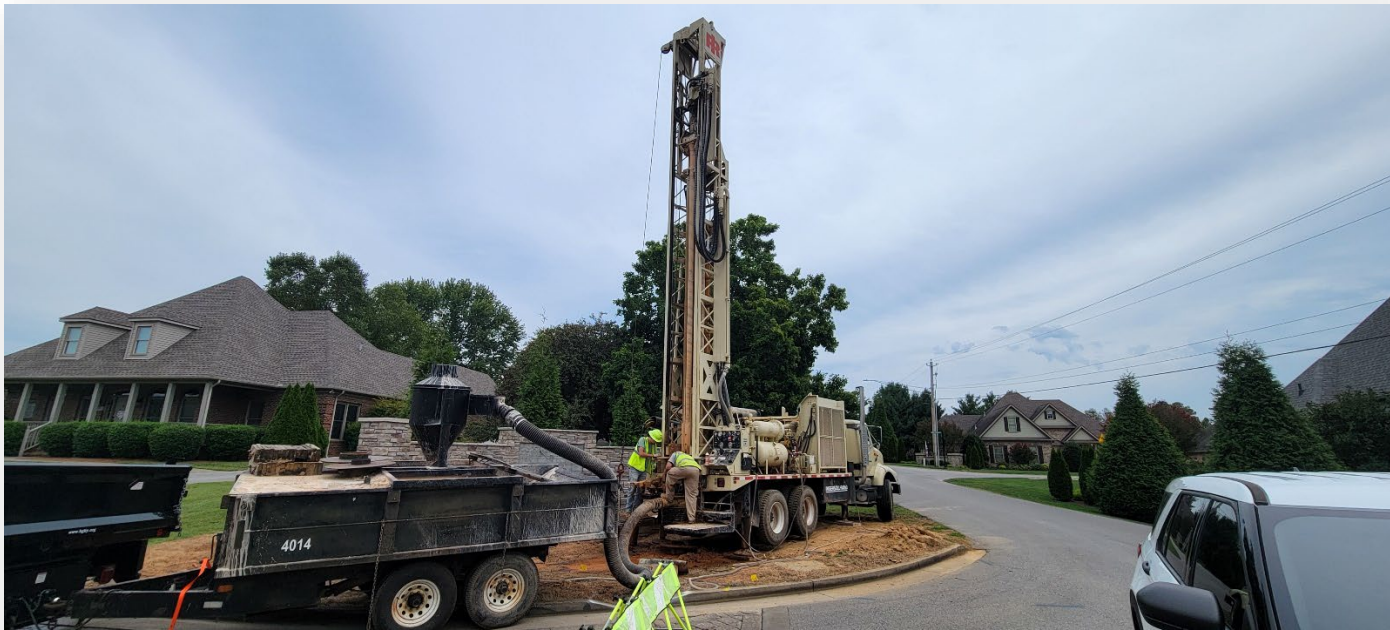
Figure 4- Crew leader Josh Miller (Right) and Operations Maintenance Technician I Zane Ward (Left) install a stormwater drywell on Talbot Drive. The well was tested with 400 gallons of water and functioned as designed (4 September)
