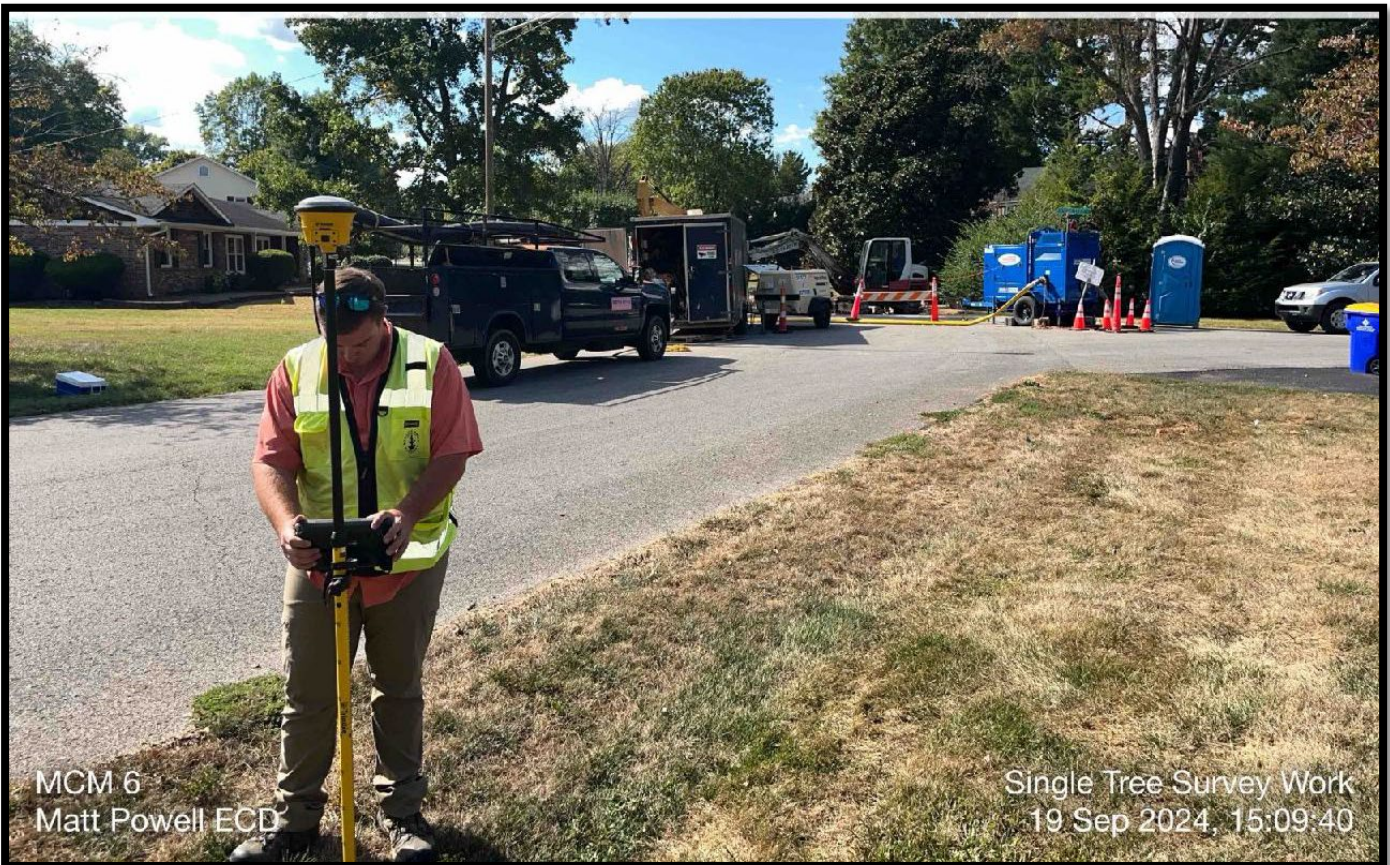
Figure 6-Construction Coordinator II Tyler Phelps assists with survey work for the sinkhole repair on Single Tree Court (19 September)
