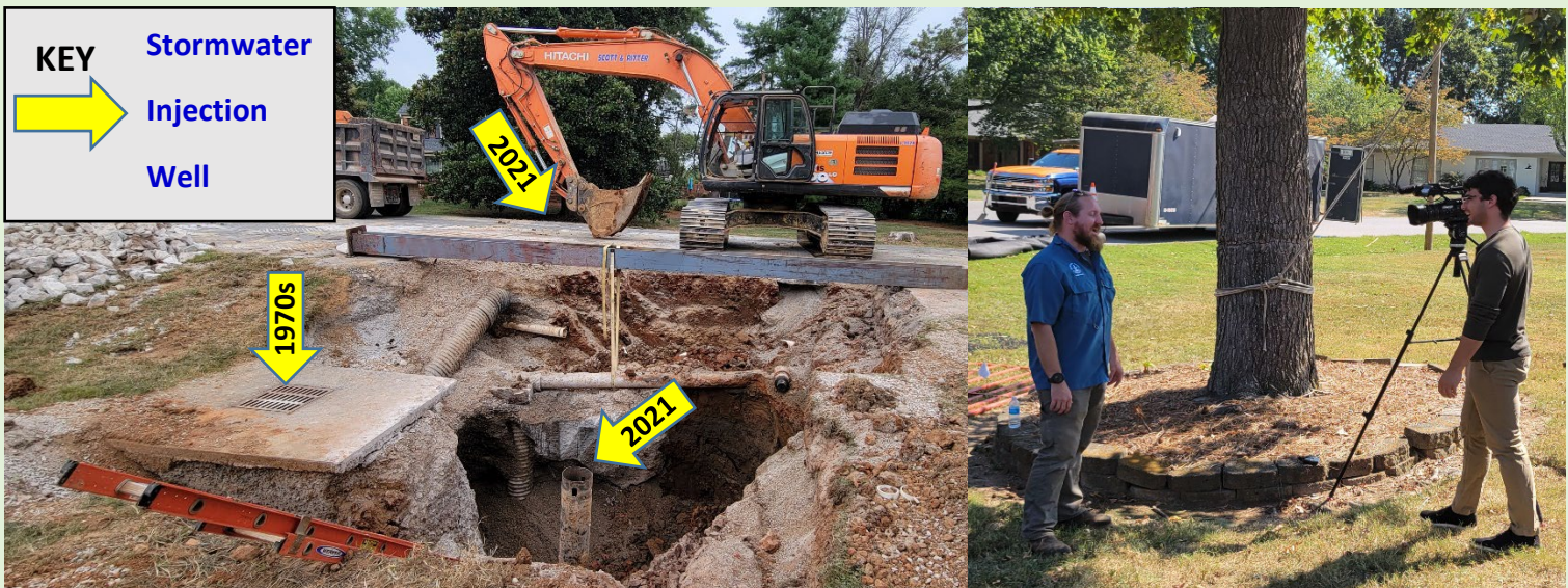
Figure 1- City Geologist Nick Lawhon led the sinkhole repair on Single Tree Way. He also explained basic karst features and sinkhole remediation techniques to the press. (11 September). Major sinkhole repairs were completed by 30 September.
